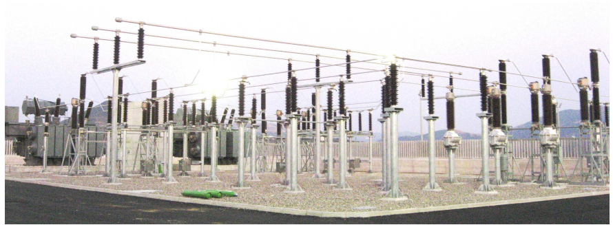
150kV Wind Farm Substation
