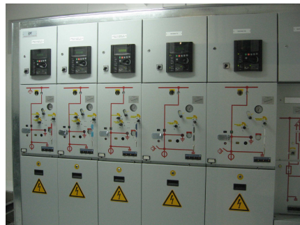
30 kV Switchgears in Subst.
