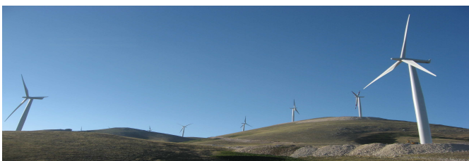
San Gregorio Magno wind farm
