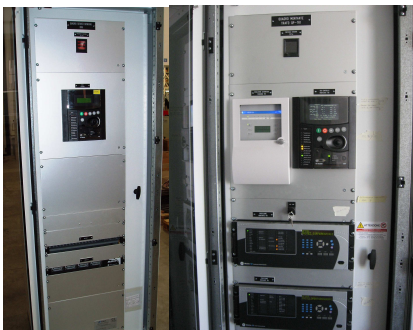
Protection Control Panel
