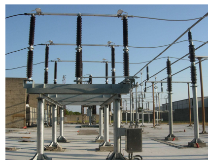
Detail of the Disconnecter-switch
