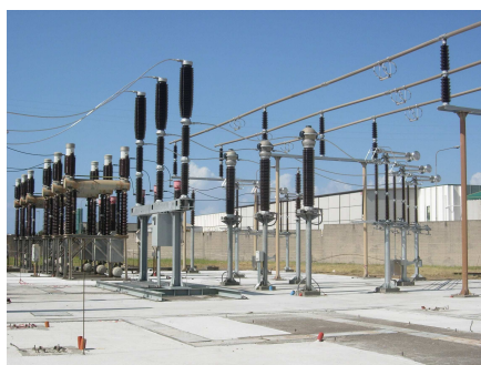
220kV BUSBAR System
