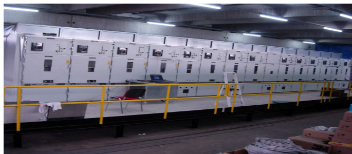
12 kV "C" Cabinet Metal Clad
