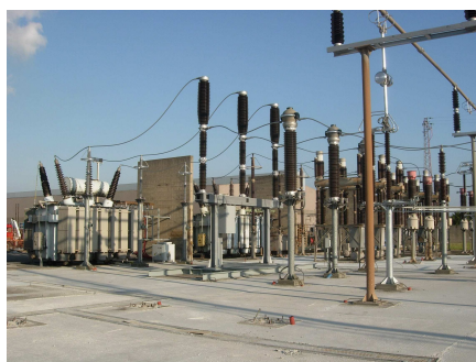
Transformer feeder Bays
