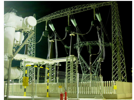
380 kV GIS conn. To 380kV line
