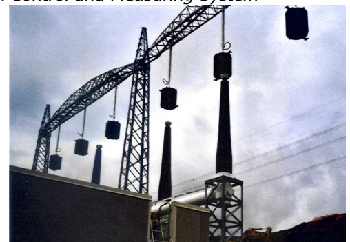
Scandale-Rizziconi 380kV Bays
