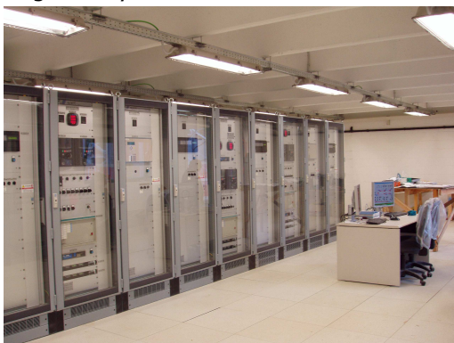
Control Room of Magisano Substation
