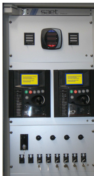
Bay Control Unit
