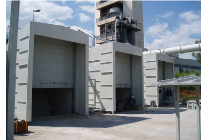
Receiving Bays for truck interface
