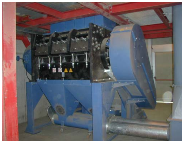
Photo of a mill (CdR Milling zone)
