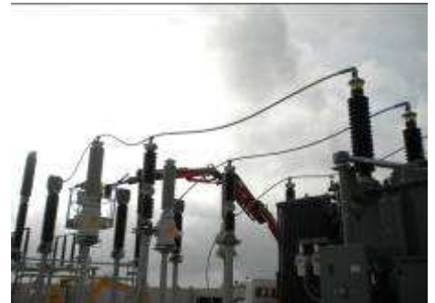
HV equipment assembly
