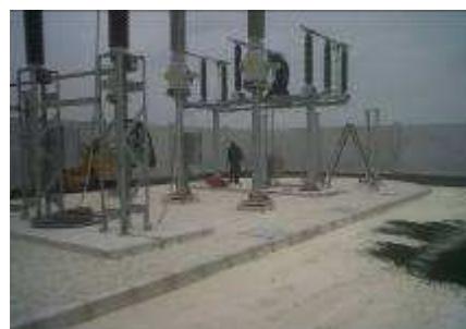
View of the HV Substation
