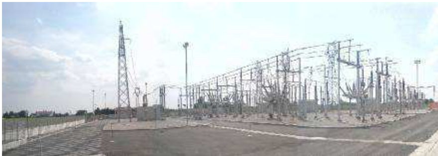
Wide view of TERNA Substation
