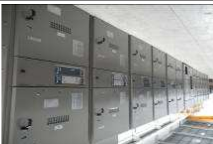
MV panel divided in two levels
