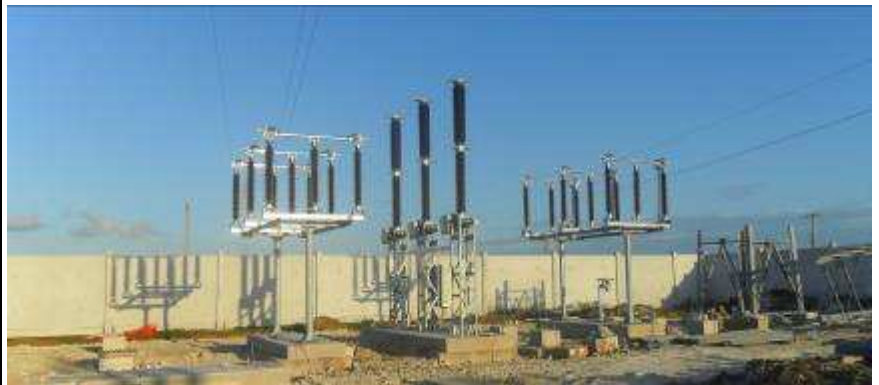
HV equipment assembly
