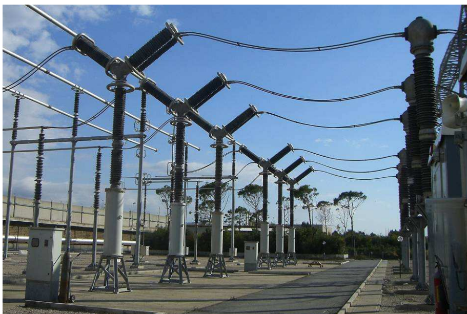
View of the substation
