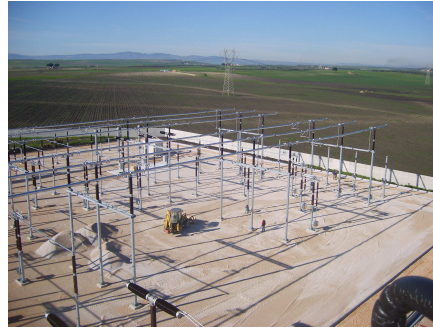
Aerial view 400kV double busbar
