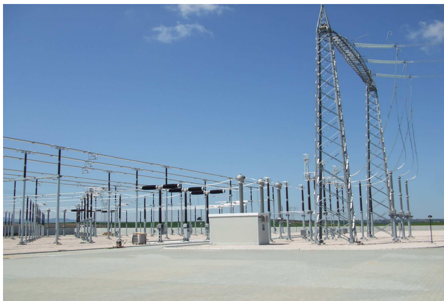
Incoming HV line bay from ENPLUS Power Plant
