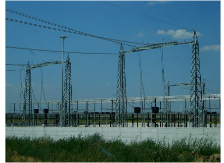
Incoming HV line
