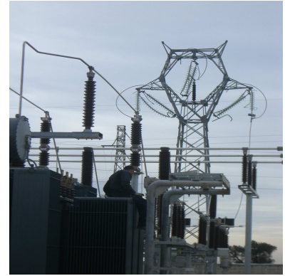
HV bay from transformer to OHL
