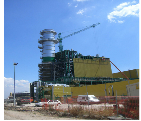
Power Plant during commissioning
