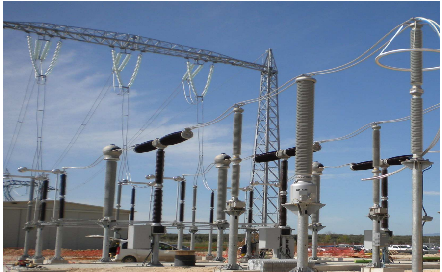
View of the Substation
