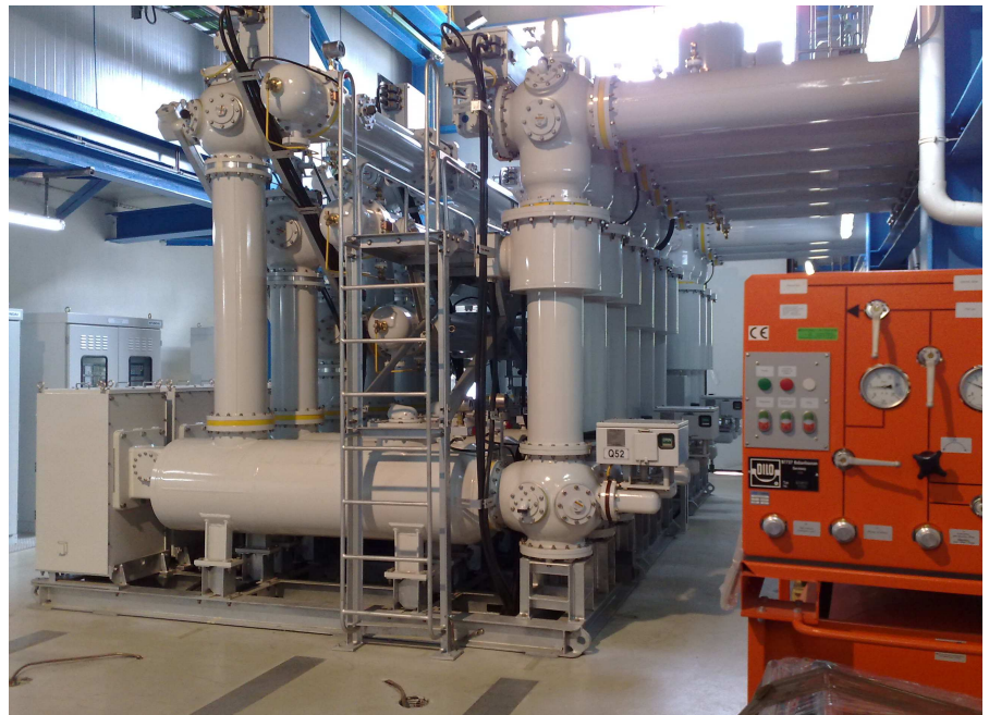
150kV GIS: the 3 bays and the bus duct towards external transformer
