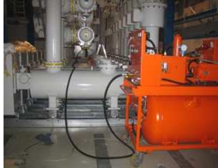
Gas filling activities
