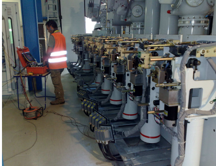
Timing test of GIS circuit breaker
