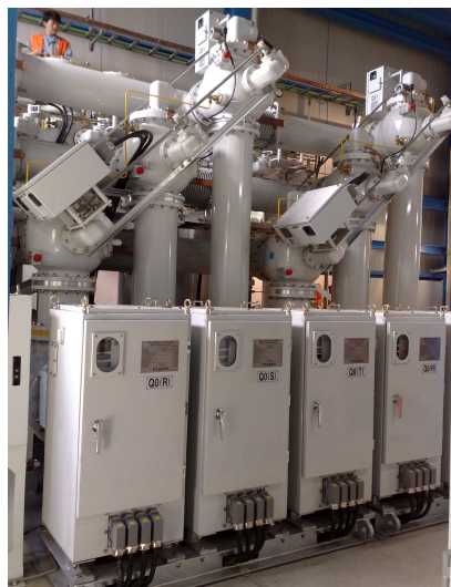
Motor drives of 150kV GIS circuit breaker
